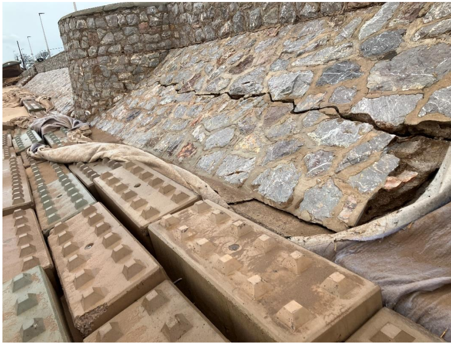
Image 1.5. Wall damage and temporary repairs.
